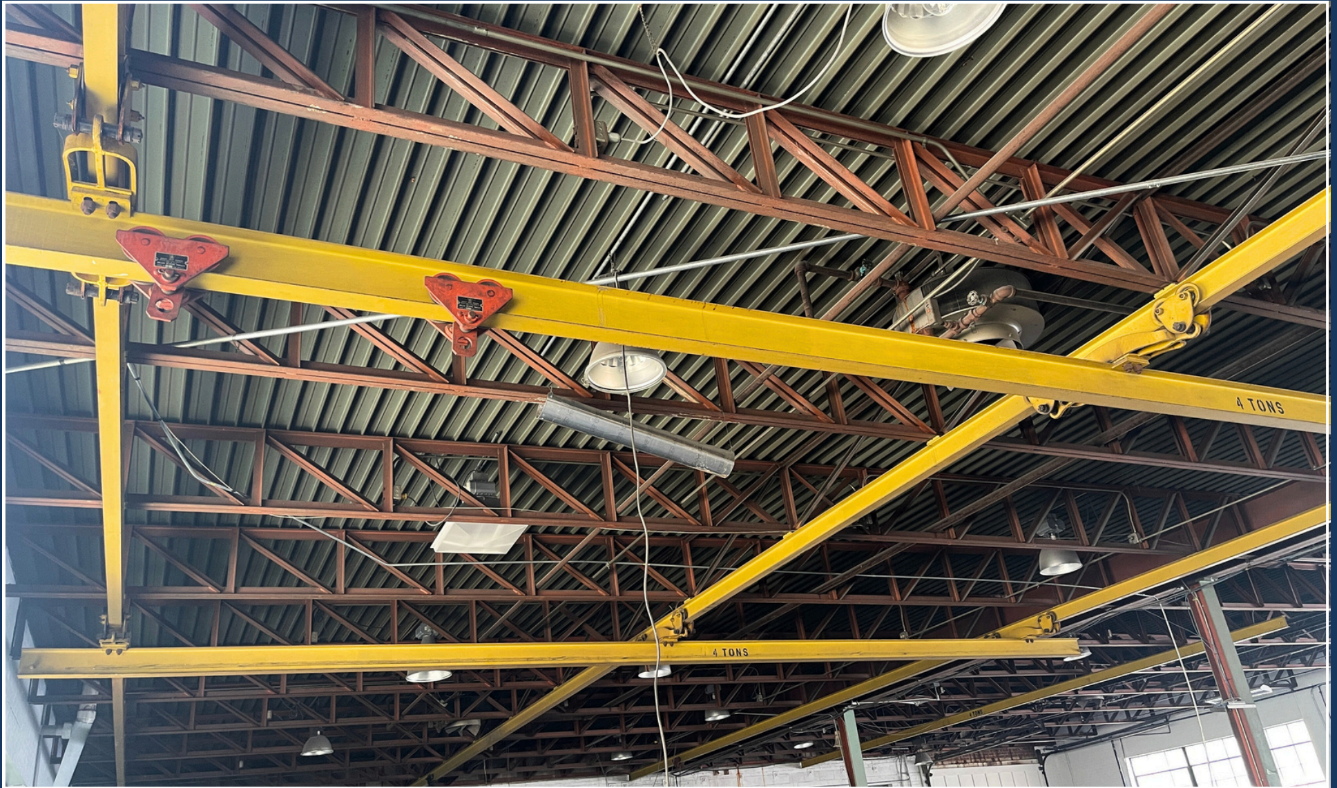
Warehouse with 4 Ton Overhead Bridge Cranes
